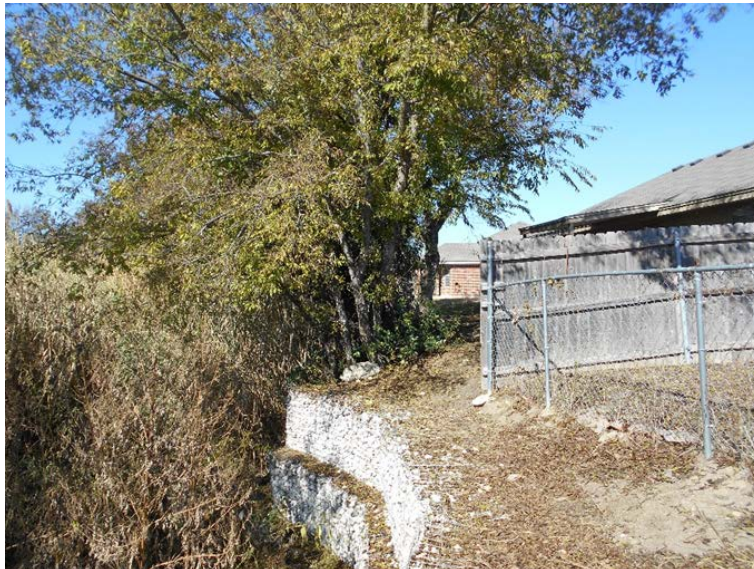
A look at the erosion at the City's drainage easement.
