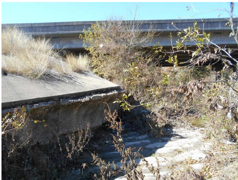
The downstream bridge abutment for the Roy Reynolds Bridge. Nolan Creek is eroding/undermining the concrete abutment.
