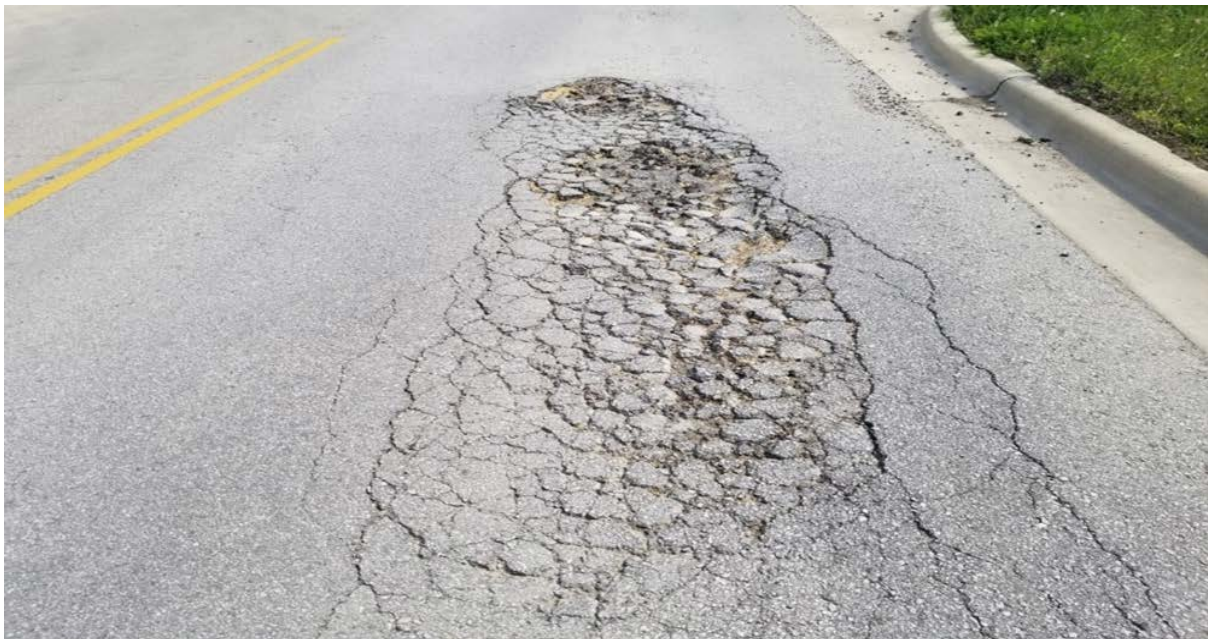
An example of damage from Winter Storm Uri.
