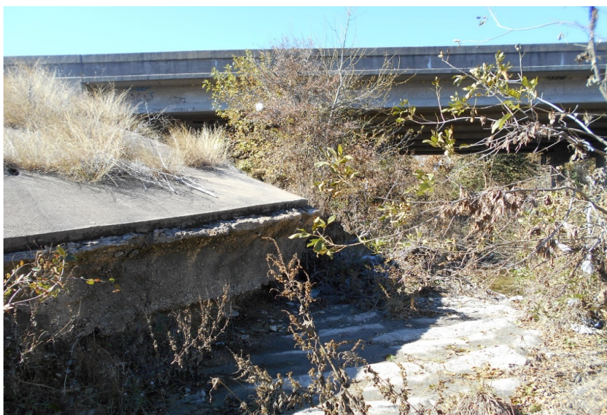
The downstream bridge abutment for the Roy Reynolds Bridge. Nolan Creek is eroding/undermining the concrete abutment.
